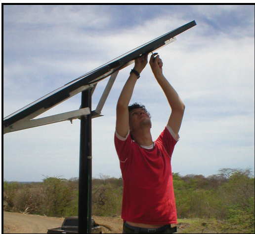
Kevin Keefe, a 2005 ETHOS volunteer installs photo-voltaic panels in El Transito, Nicaragua
